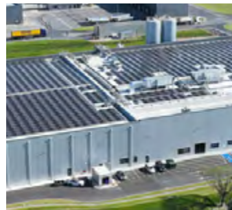
Solar panel array on the roof of the plant
